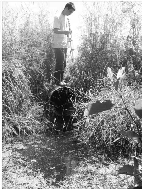
Summer student Brandon Rushton surveys a culvert as part of the Adopt-a-stream program with Friends of the Pugwash Estuary.
