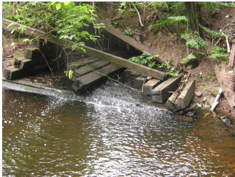
Featured Photo: This is a picture of a fallen culvert on the Canfield Brook.
